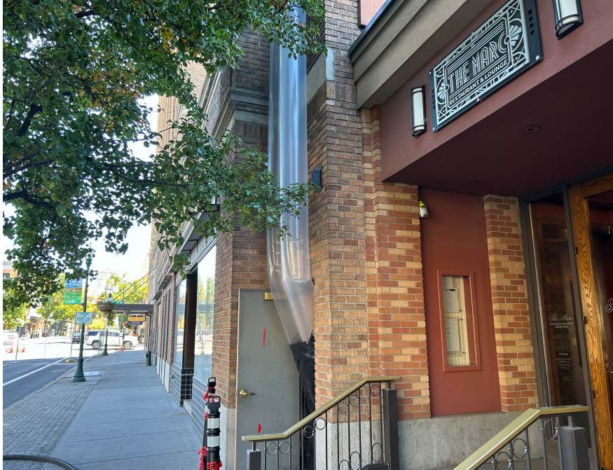
Ventilation exiting the building and routed to the roof for exhaust.
