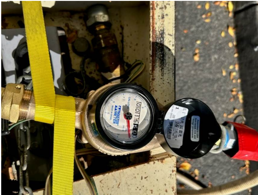
Processed water discharge to the municipal wastewater system being metered.
